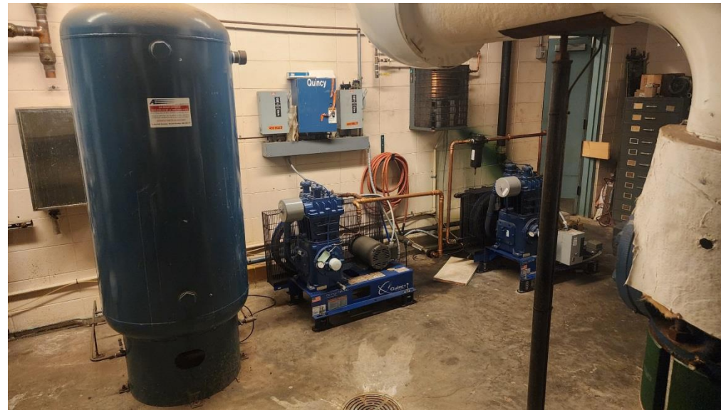
Compressor and Air Tank
