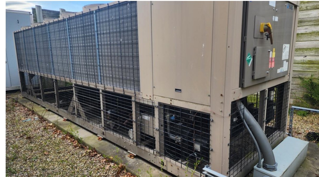
High School Chiller
